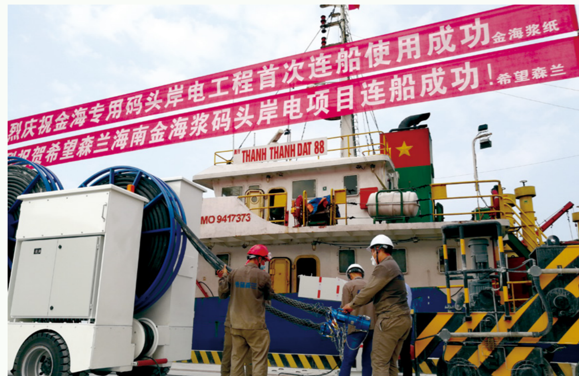
The shore power project at Hainan Jinhai Pulp & Paper's exclusive terminal was successfully commissioned for the first time
